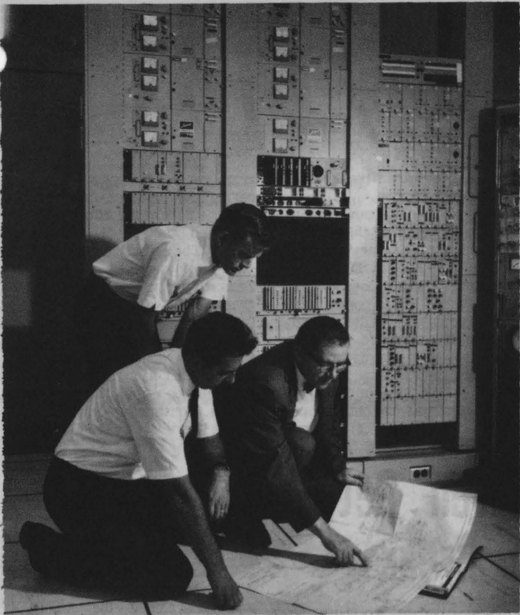
CHECK THIS - The Lenkurt 76C Microwave Radio installation at the Range Control Center is shown in the background as Bob Canavero, Lenkurt installation supervisor, left kneeling, and Chuck Parker, WSMR program manager for Lenkurt, examine over-all system plans. Ray McPherson, White Sands test technician, is pictured standing. (U.S. Army Photo by Robin Broun)
